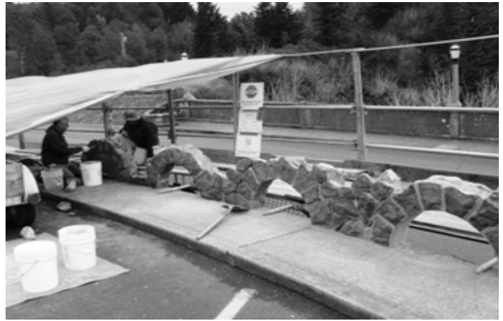
Photo courtesy of Pioneer Waterproofing
